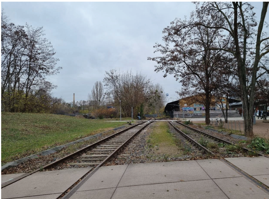
Pic 48 Old railroad with new concrete path construction in Park am Gleisdreieck (Shahrokhi,2022).
