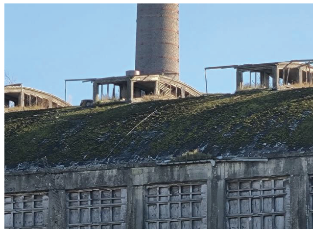
Pic 38 Moos on the concrete roofs (Shahrokhi,2021).
