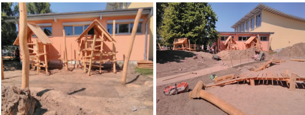
Figure 3.4: Construction site set up outside the courtyard of the kindergarten (Source: Personal archive)
