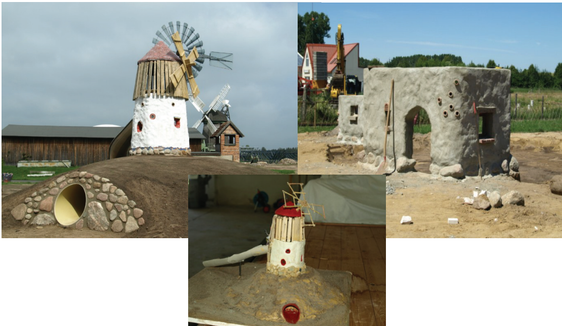
Figure K : Stages of windmill construction ( Final stage, Initial manufacturing stage, a model of the windmill of Alt Schwerin Playground (Source: From the Personal archive of Fiedler Sabine)
