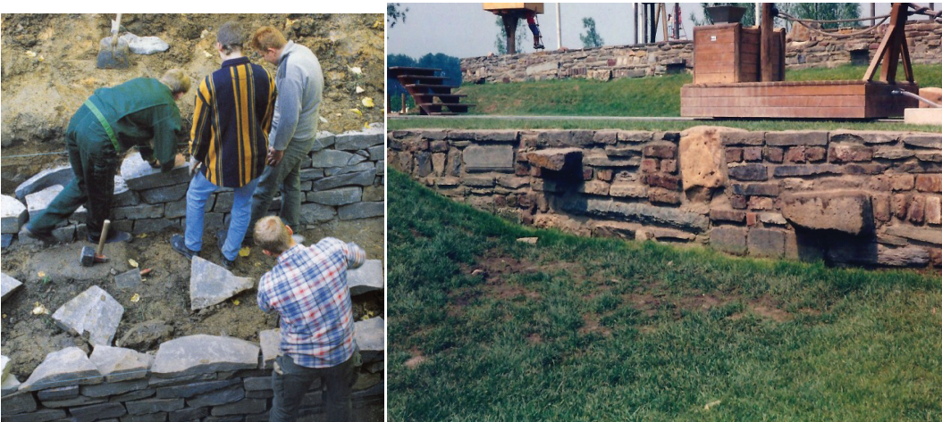
Figure Q: Details of the construction, before and after (Source: Personal archive of Oyen Thomas)
