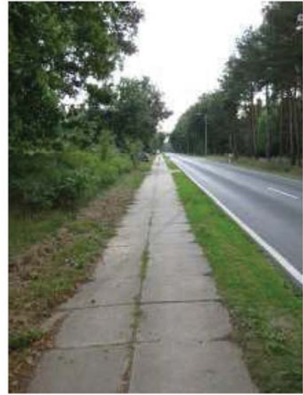
Abb. 9: Betonplatten in Hammer
